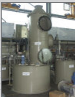
Washing system for purification of exhaust air
