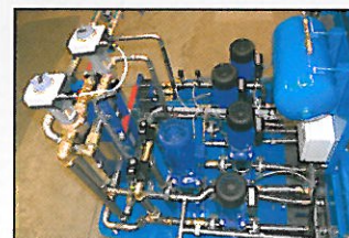
WATER COOLING SYSTEM
