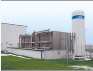
Industrial water cooling
