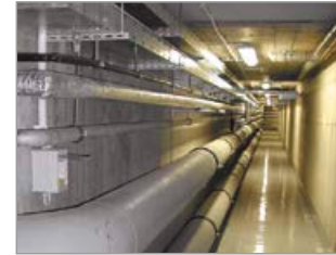
Underfloor supply pipes
